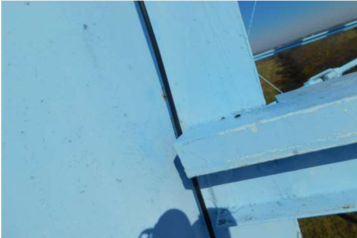
Photo shows the condition of the strut end connections. The strut ends have been sealed welded and appear to be in good condition.
