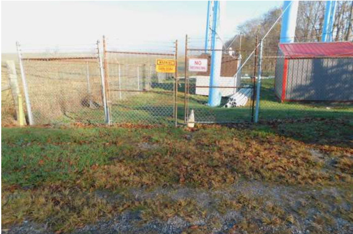
Notice the site is marked to identify the storage tank site security status.
